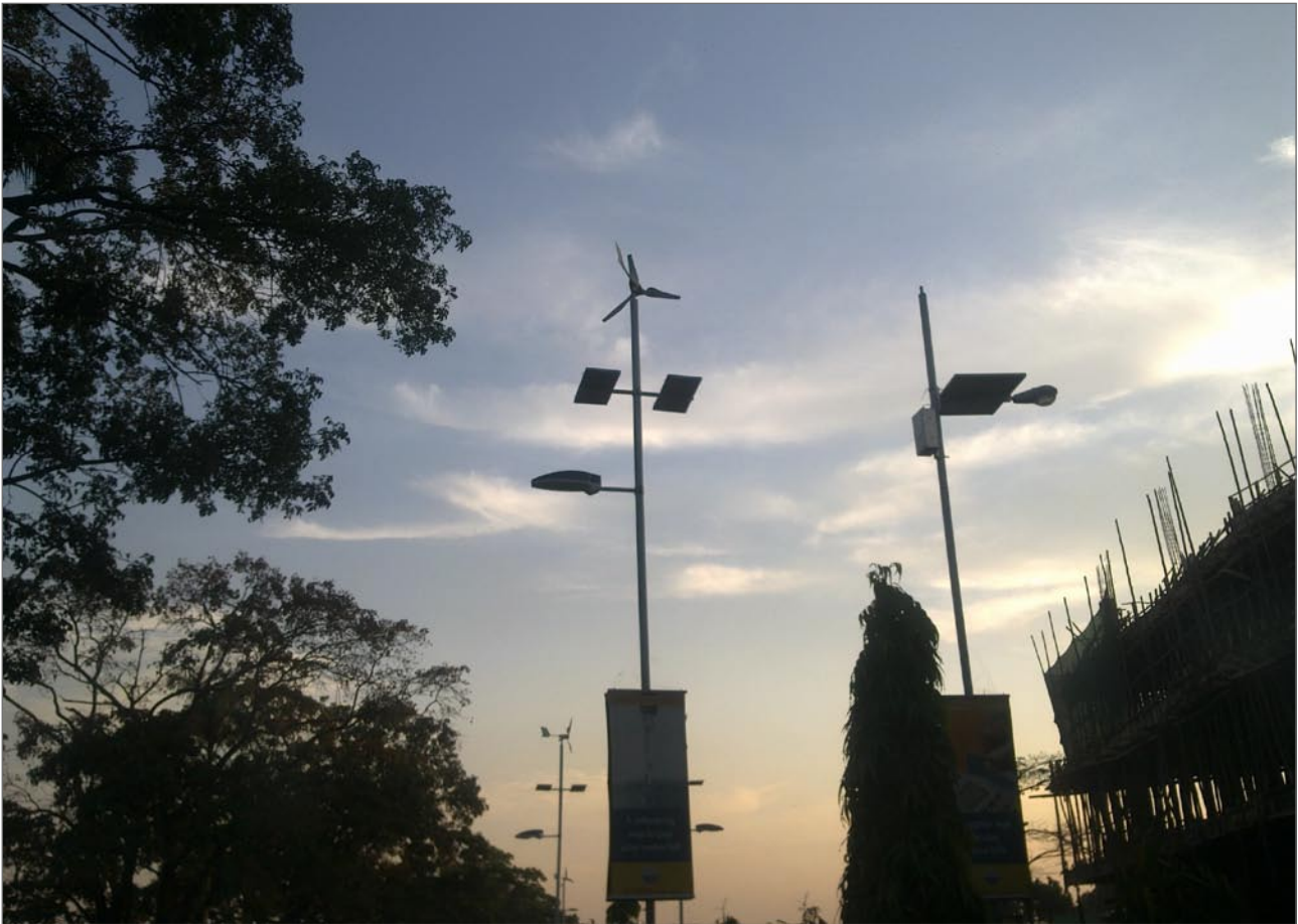
Solar street lights installed along Entebbe Road in the capital city Kampala.
